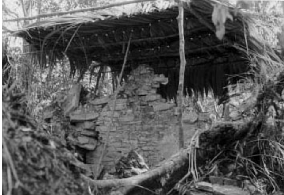
Figure 9: Protective shelter constructed over southern wall of central room, Structure 1, La Pasadita.
