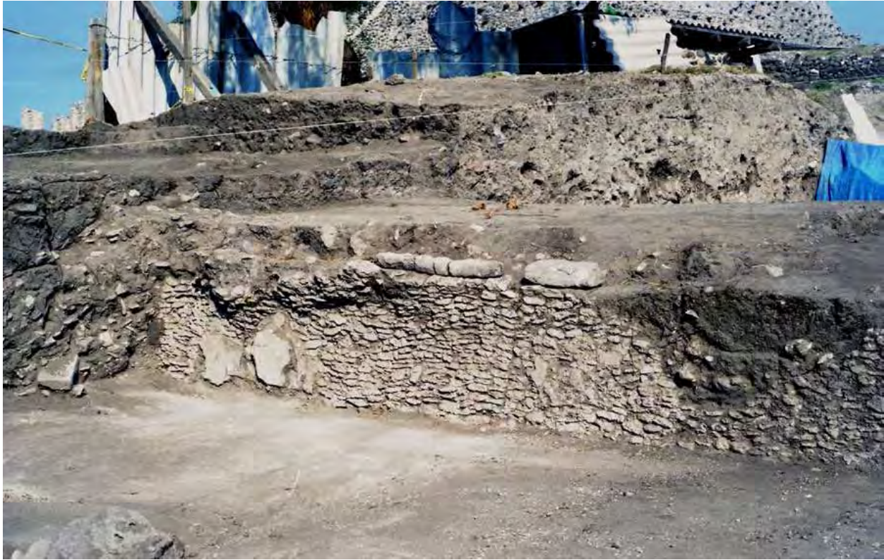
Figure 22. State of conservation of the wall made of slats of "small stone" at the structure's southwest end. See the partial height bordered by quarry stone cornices.
