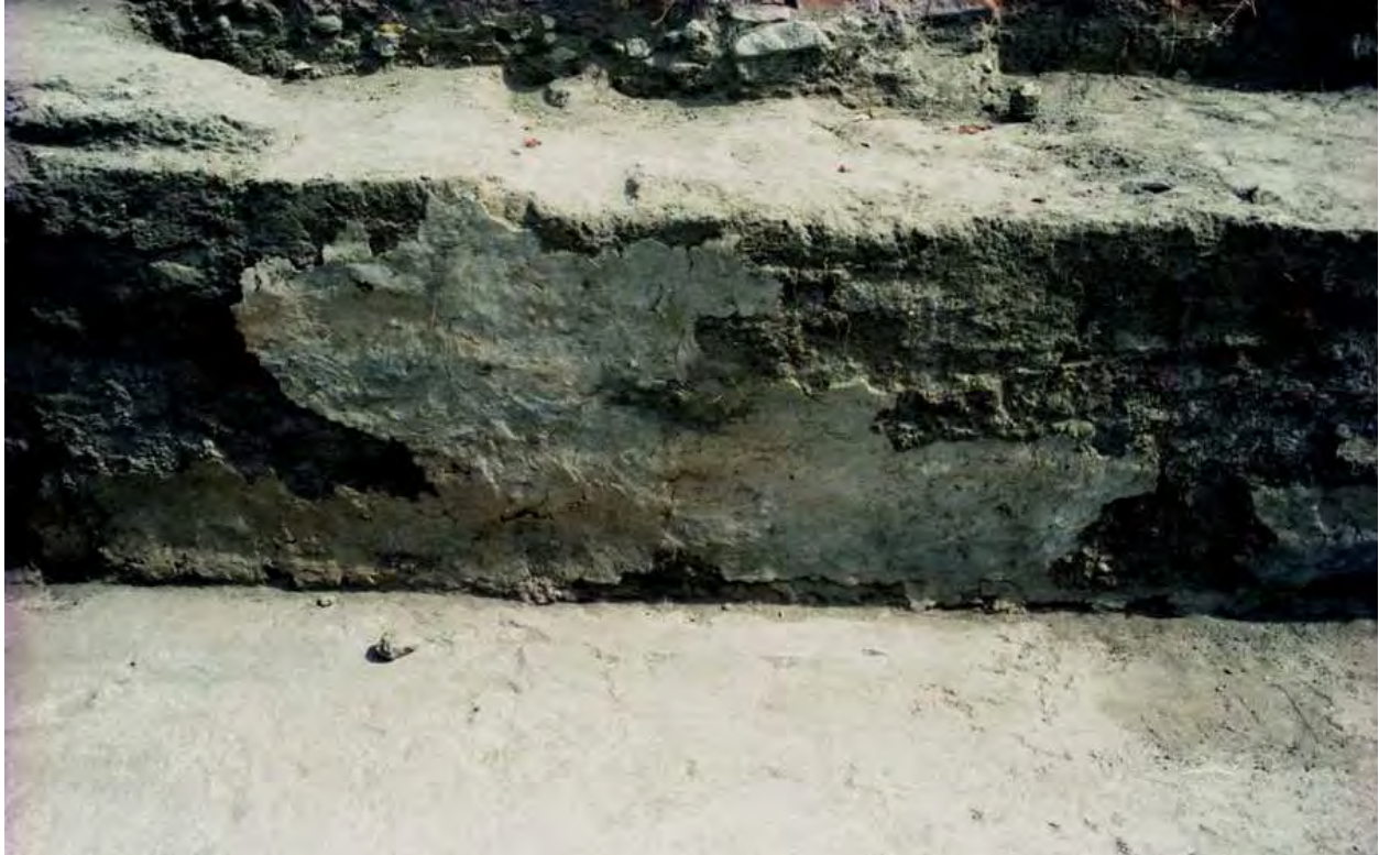
Figure 17. State of conservation of the adobe walls, in which we see the core made of blocks covered with a coat of clay. These rise directly from the floors, with no evidence of banquettes.
