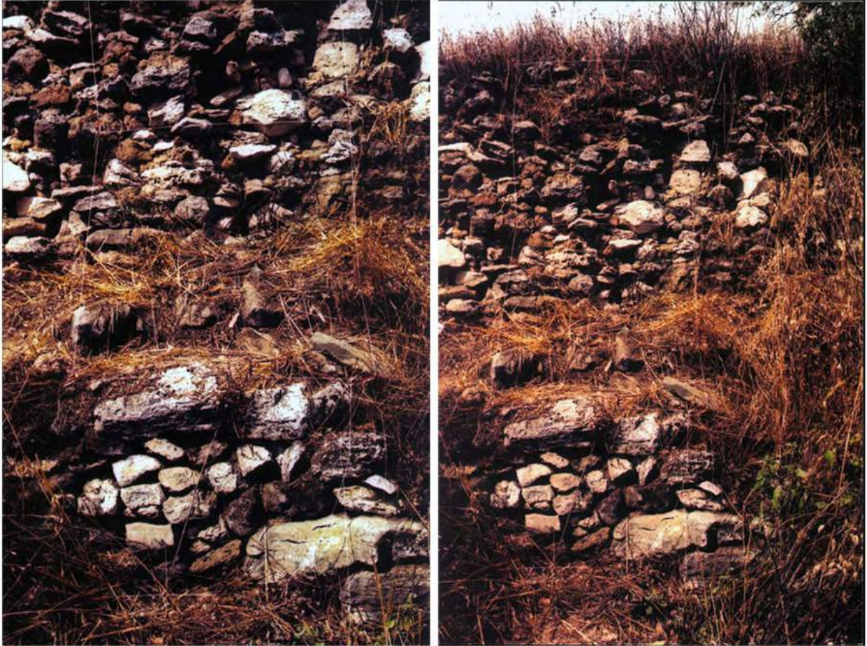
Figure 15. Plaza 1 South Retaining Wall (Rubble Core Exposed).
