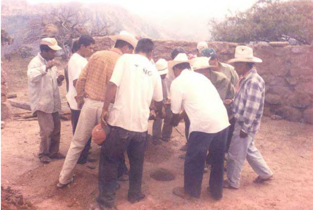
Figure 26. Putting the temple's central post in place. Prayers and offerings before the post is erected in the posthole. Photo provided by Mr. Pablo Muñoz.
